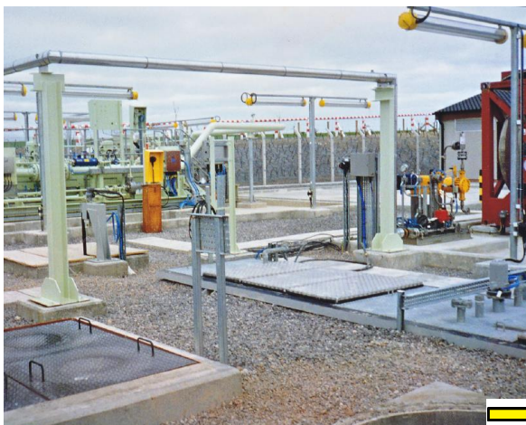
Monitoring in an Unmanned Pumping Station
