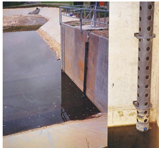
ID-221 Monitoring Runoff from a Highway Junction
