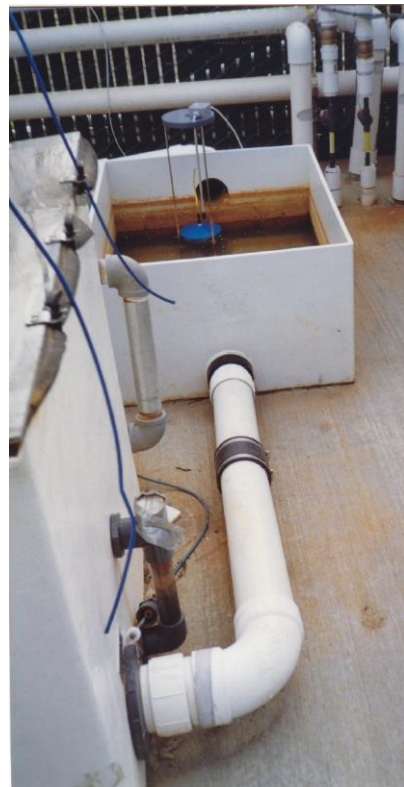
ID-223/500 in a Settling Tank
